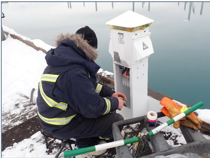
Puffin terminating conductors on lugs in float power pedestal
