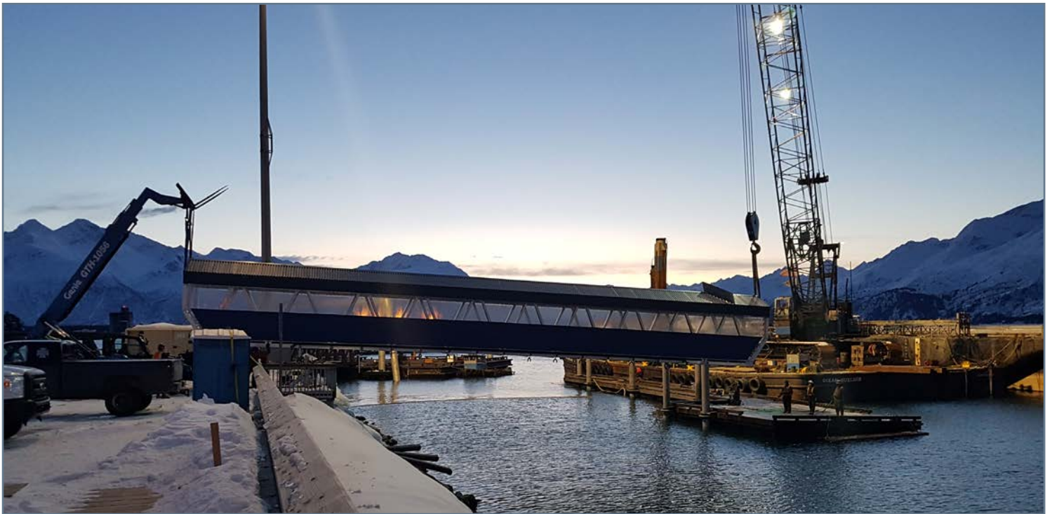
Lifting Gangway 3 into position on shore lug (left) and float landing plate
