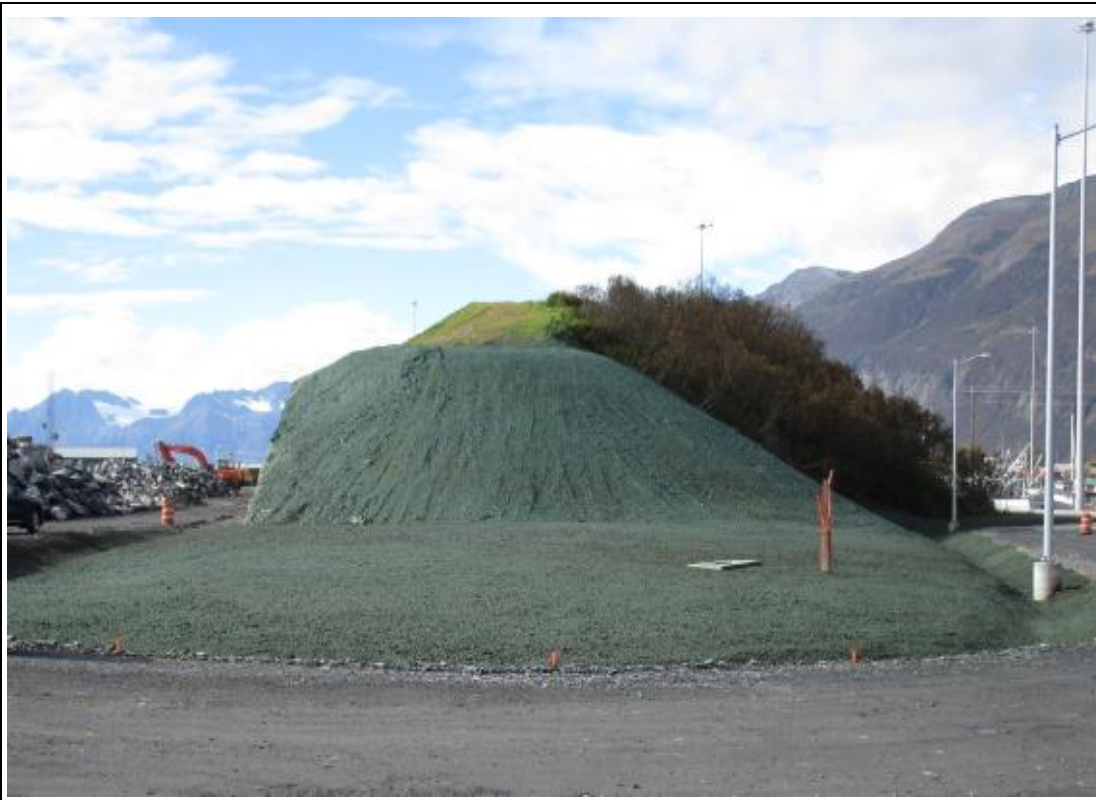
Topsoil hydroseeded at East end of Hotel Hill; street lights installed along East Access
