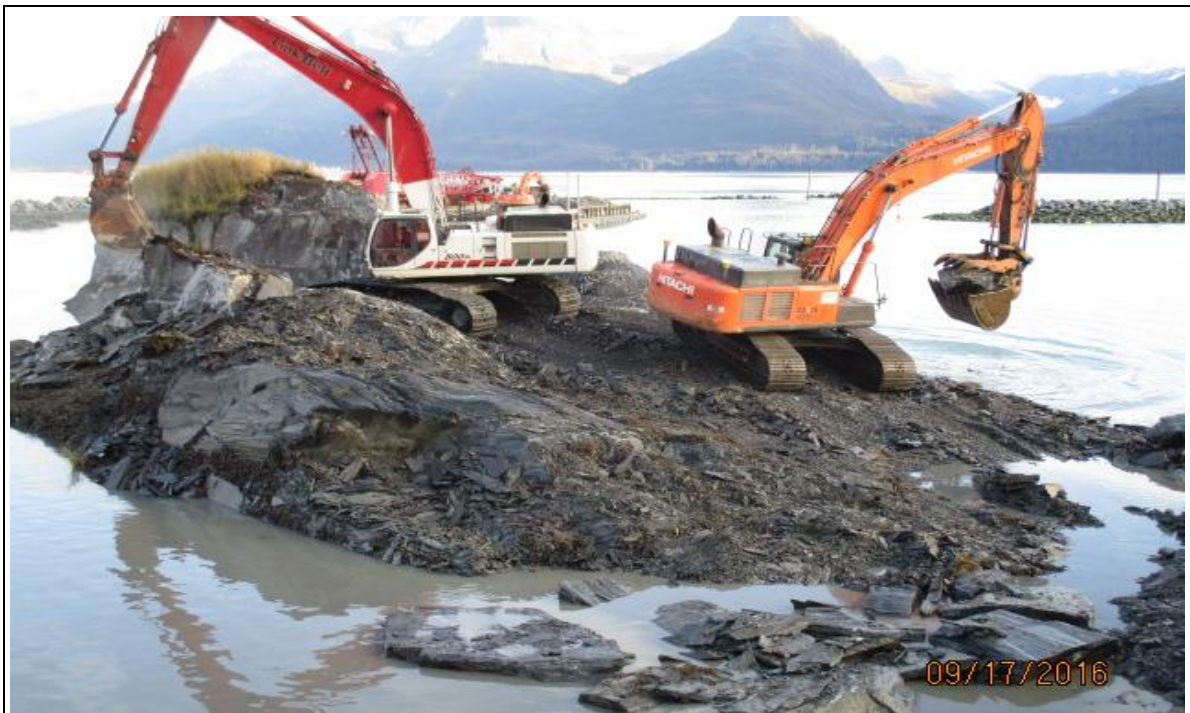
Hoe with rock bucket (left) breaks bedrock while hoe with “thumb” places large rocks for future drill pad
