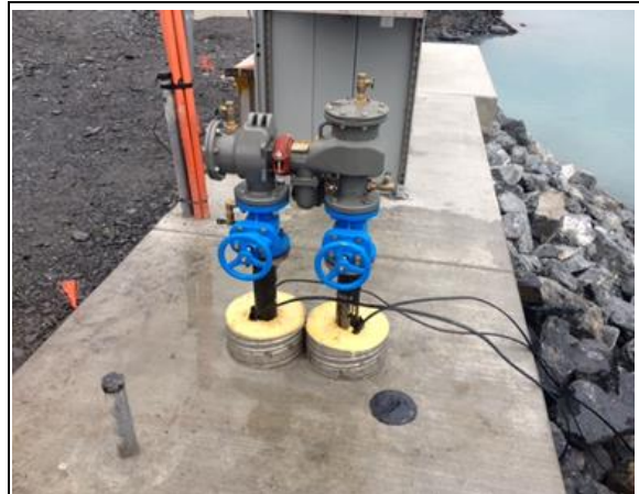
Installed backflow preventer (BFP) at Ramp #3
