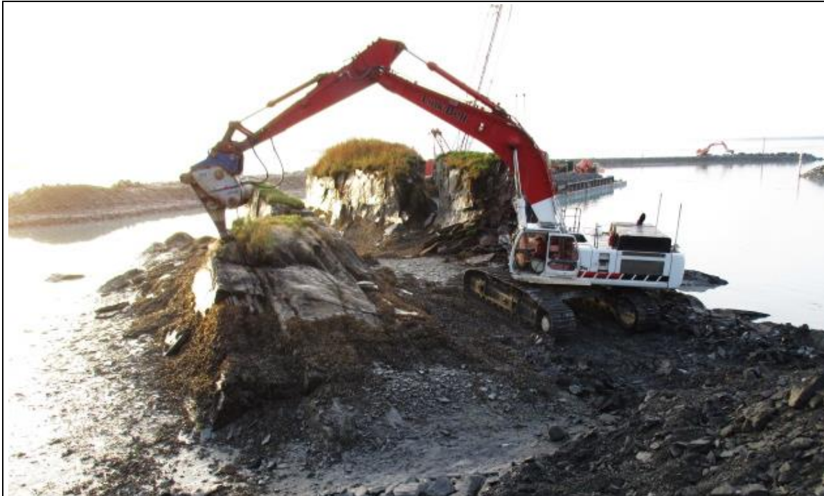
Testing Xcentric Ripper ability to break bedrock at rock outcrops in proposed Drive-Down Float basin
