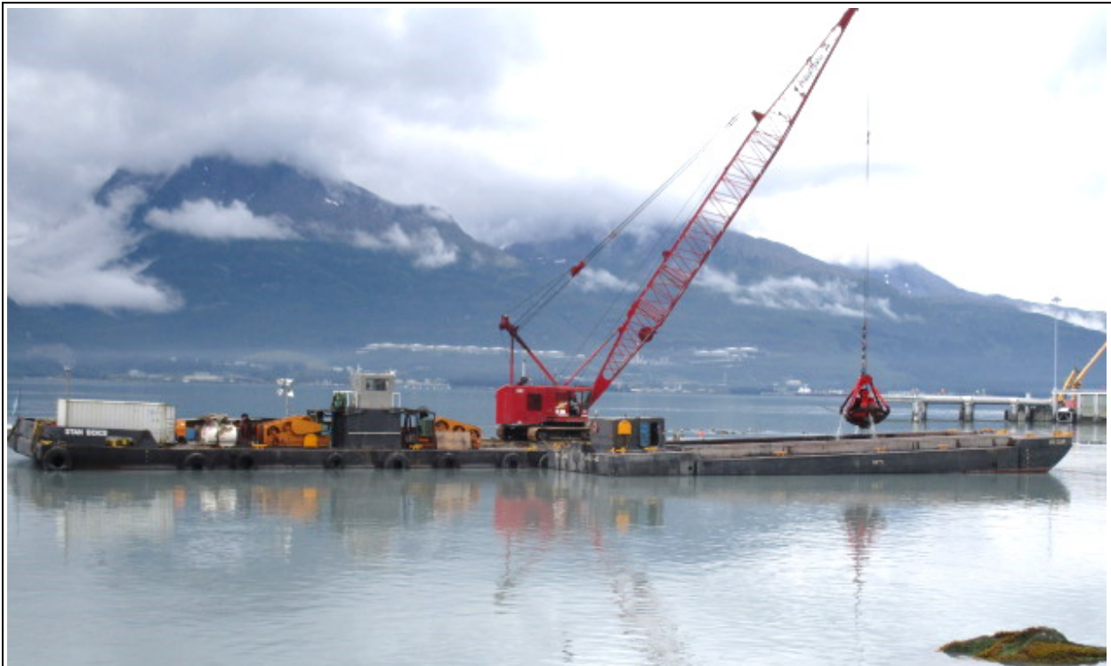
Western Marine continues dredging sediment to create the maneuvering channel and basin for the new harbor
