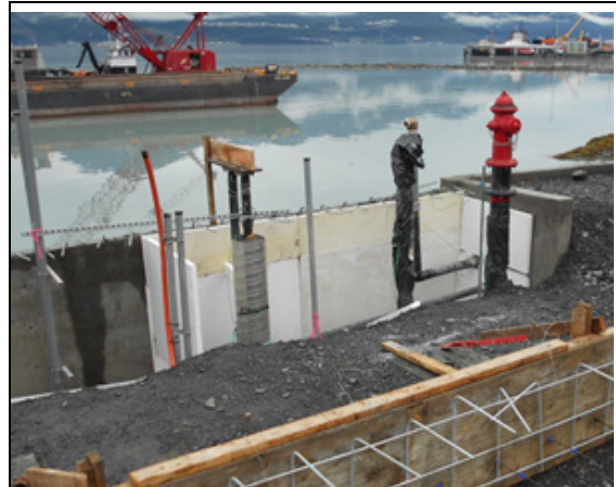
Insulating backflow preventer (BFP) foundation
