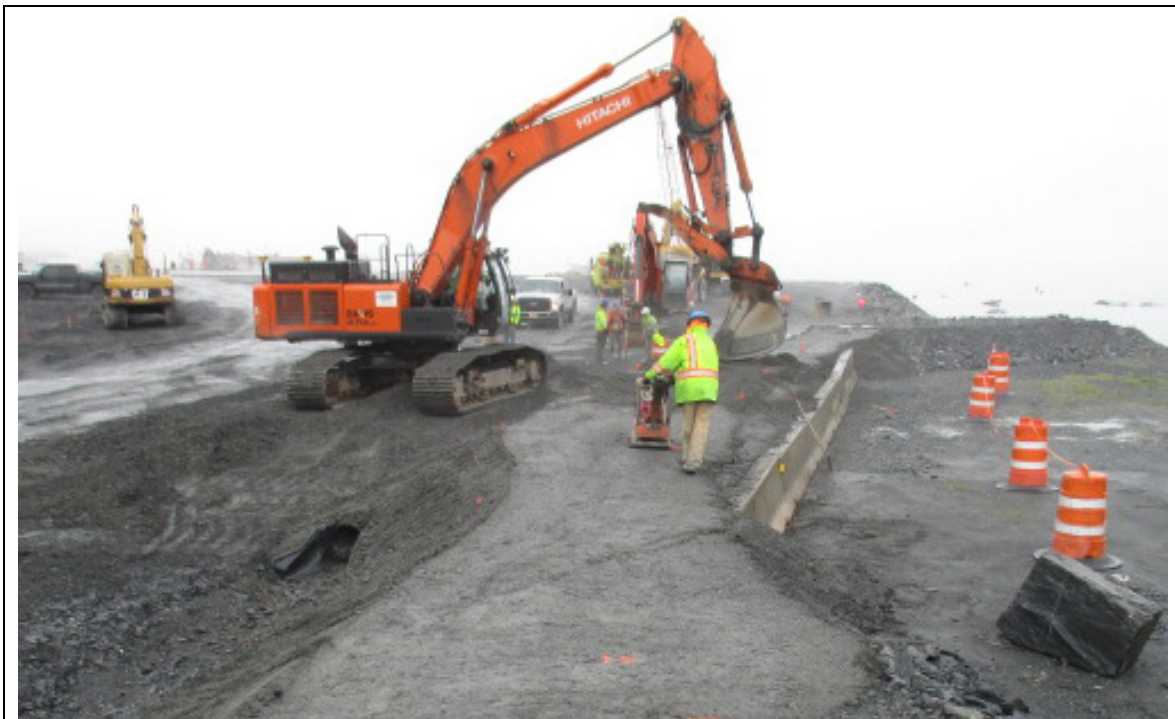
Compacting fill for a berm between the West Access and barricades placed along SERVS property
