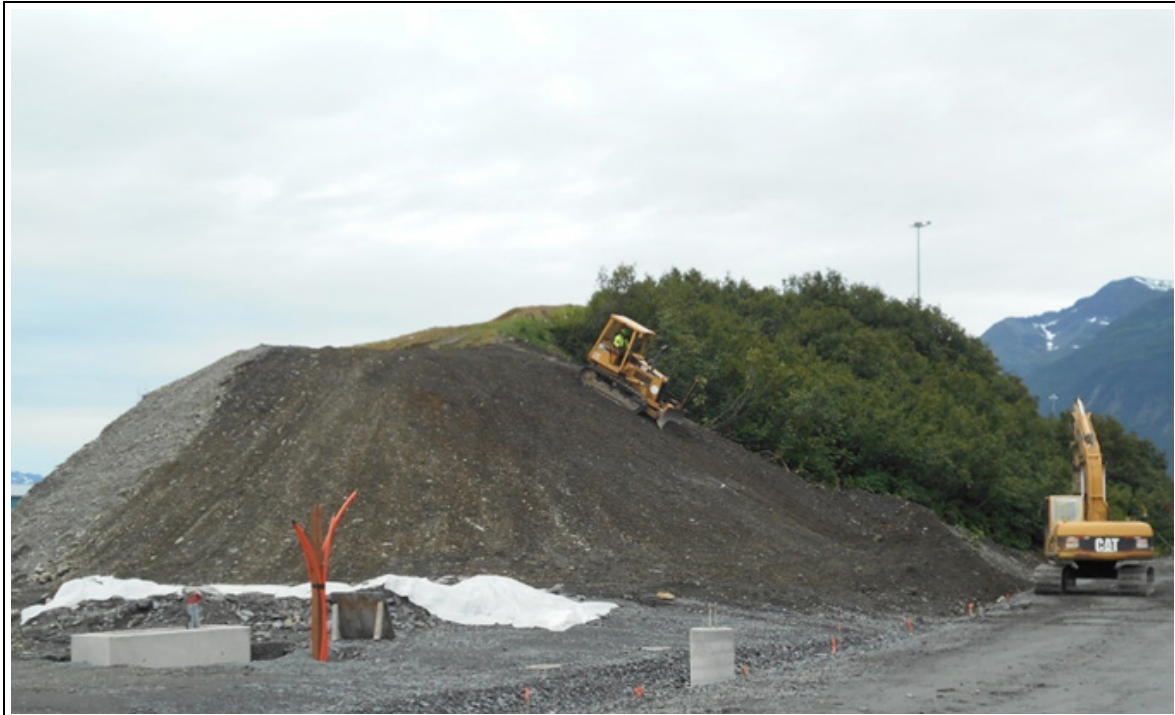
The slope at the east end of Hotel Hill was final graded for seeding
