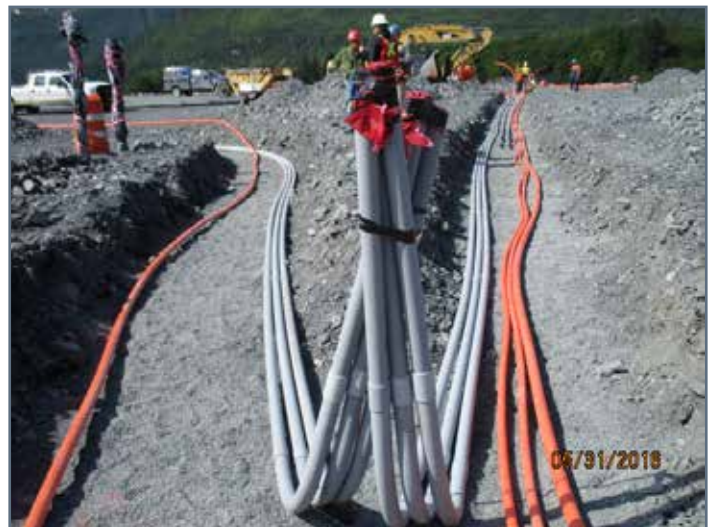
Site electrical and utility conduit with risers in common trench
