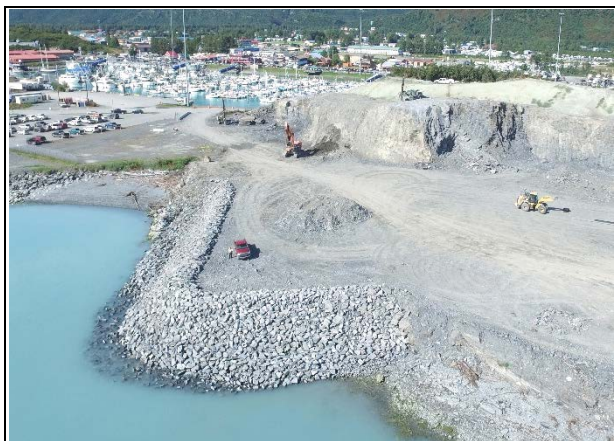
Temporary riprap protects new launch ramp area until Corps of Engineers' contractor constructs the breakwater
