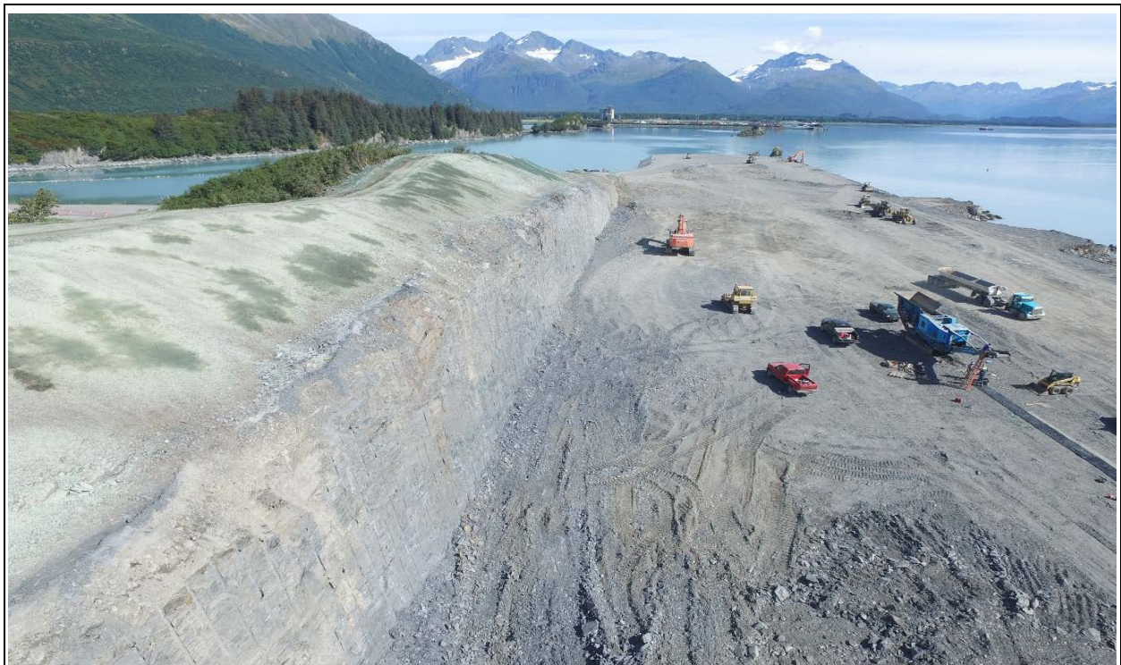
Upper 2:1 slope (left) has topsoil and hydroseed. Finished bedrock cut (left of center) is 1H:4V. Most of the right side has been excavated and rough-graded 2' below finished surface. East fill is at far end. (J. Talbott, COV)
