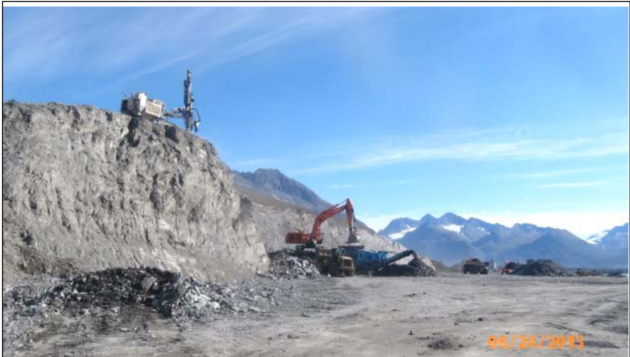
View East. Drilling, shooting and excavating bedrock in progress at NW corner of site. Excavator (center) is feeding crusher with shot rock. Right side shows the site has been excavated and fine-graded 2' below final grade/pavement.
