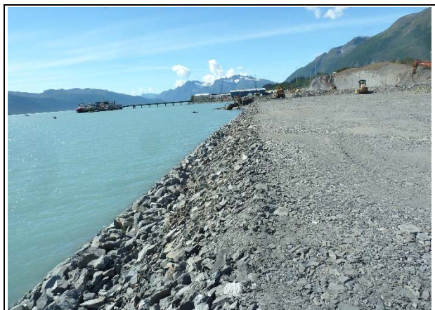
South shoulder of east fill being shaped 1½:1 before 1' layer of filter rock and 2.5' layer of riprap are placed
