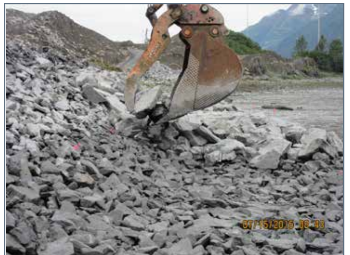
Placing riprap on filter rock at toe along north side of tidelands fill.
