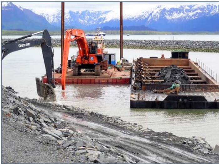
Deere 870 (at left) excavates and stages rock for EX1200 with clamshell bucket on Flexi-float barge to reach and place on dump barge
