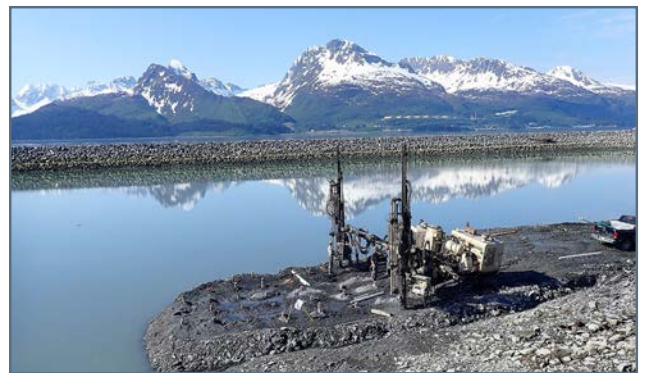
Drilling holes for blasting rock at the West part of mooring basin
