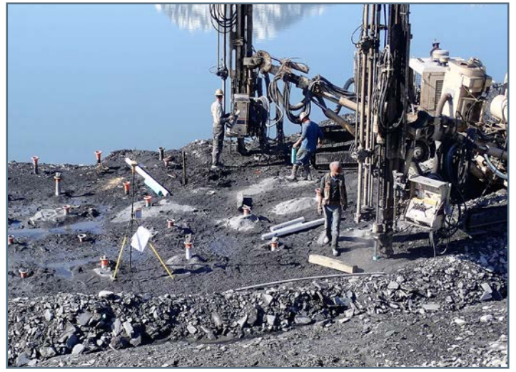
Drilling holes for blasting rock at the West part of mooring basin
