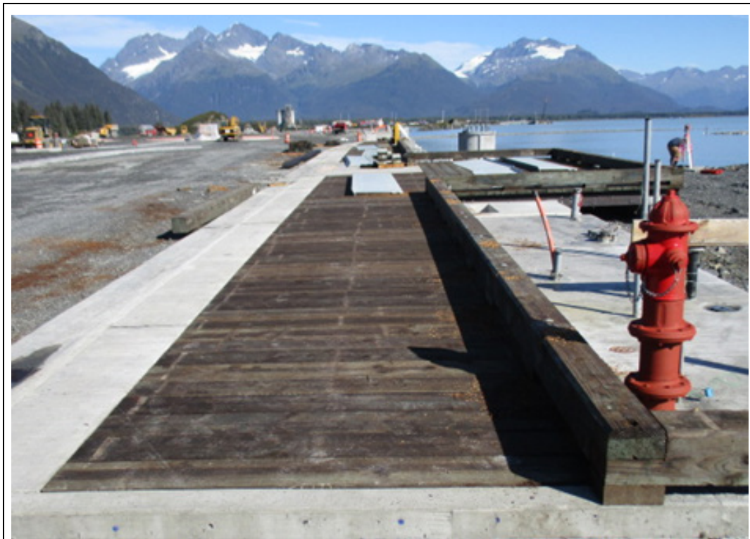
Concrete curb and sidewalk, boardwalk deck with bullrail, and concrete utility pad
