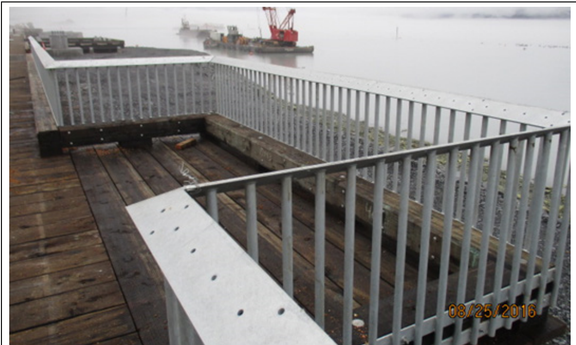
Guardrail with top plate attached to bullrail at rest area. Timber handrail will be bolted on the top plate.
